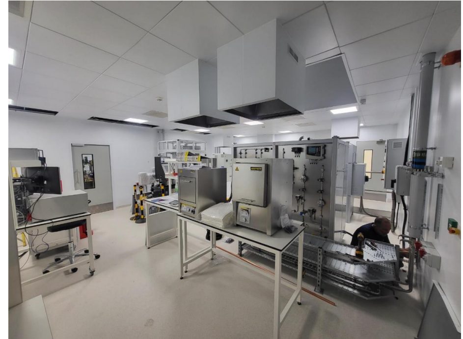
3D-printed Ceramic and Metal heat treatment facility
